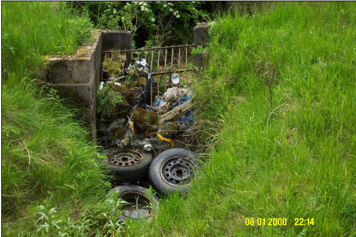
Entrance to Preston Hill culvert obstructed by debris
