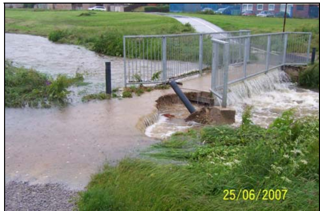
Wyke Beck flooding June 2007
