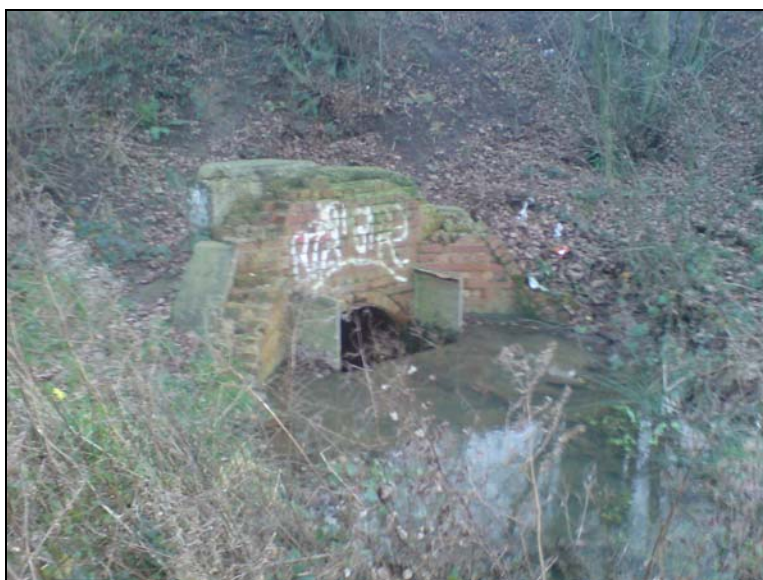
Difficult access to Stanhope Road culvert
